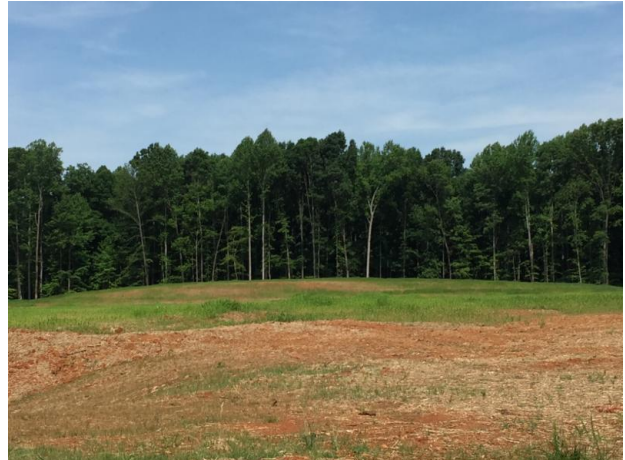
One of the recently graded lots is Lot 4, located at the end of the cul-de-sac on East London Drive. It is 24+ acres with 10 acres graded.
